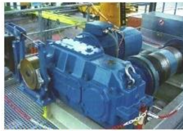
Main hoist drive 煤矿主提升机驱动
